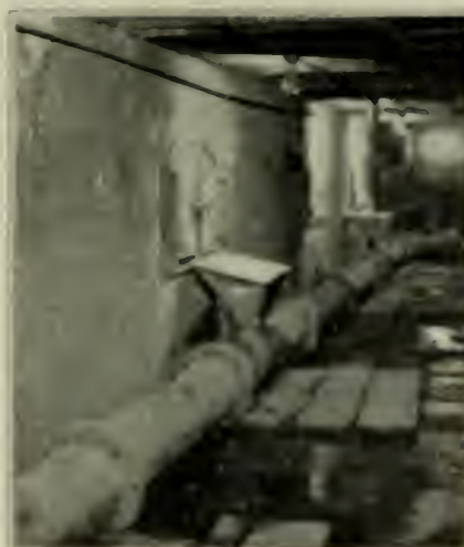
FIG. 4. CONVEYER PIPE IN TRUCK OF ASHES
